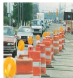
Work zone ITS
